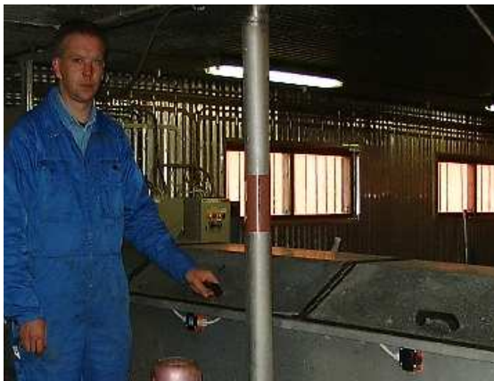
A very pleased operator, Anders Nygårds, at the Siljan RotoMaster drum thickener
